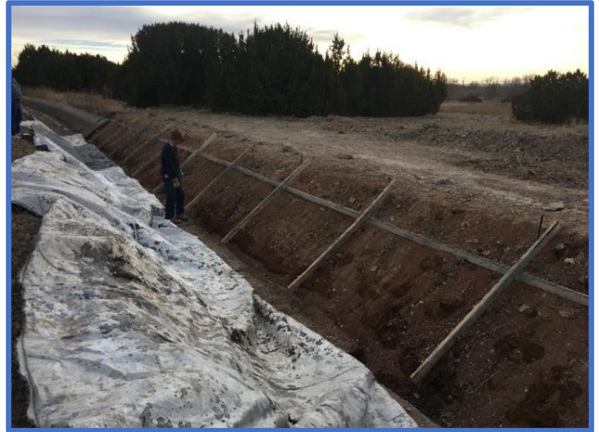
New concrete lining section forms in place. Freeze protection cover ready. March 2018.
