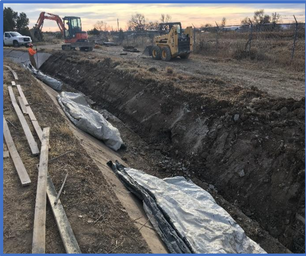
Failed canal lining sections removed. March 2018.
